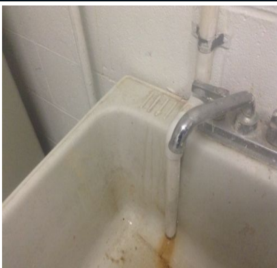
31 05-A Domestic Water - Water Supply/Pipes
