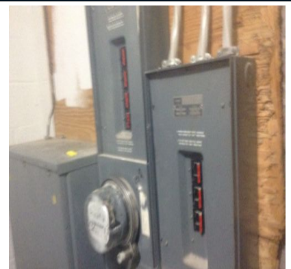
33 05-A Electrical System - Electric Panel
