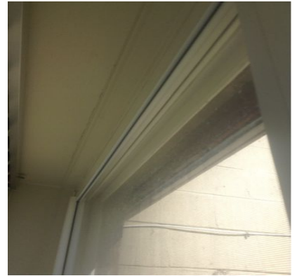
45 05-A Unit 01 Bedroom 1 - Window Seals/Sills
