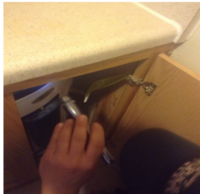
62 05-A Unit 03 Local Systems - Water Heater
