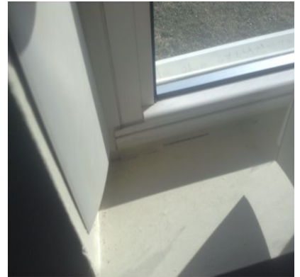
60 05-A Unit 03 Living Room - Window Seals/Sills
