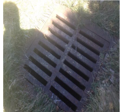
9 Site Storm Drains - Storm Drains
