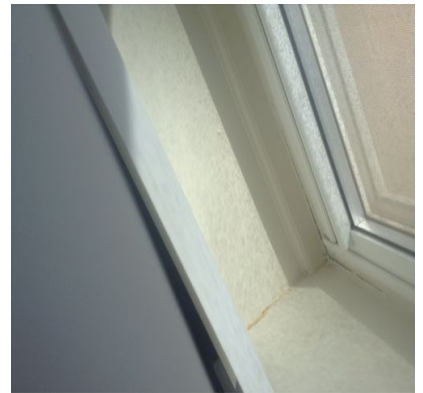
51 05-A Unit 02 Bedroom 1 - Window Seals/Sills
