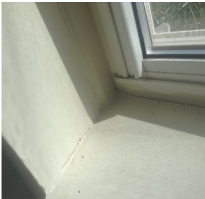
49 05-A Unit 01 Living Room - Window Seals/Sills
