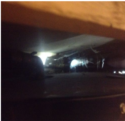
61 05-A Unit 03 Local Systems - Water Heater
