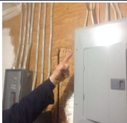
32 05-A Electrical System - Electric Panel
