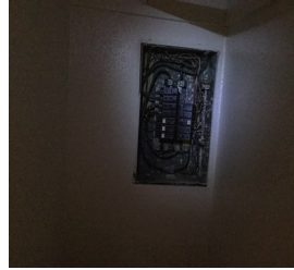
20 608 Unit 608-20 Other - Breaker Box
