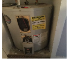
21 608 Unit 608-20 Other - Water Heater
