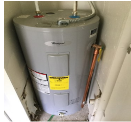
3 604 Unit 604-02 Other - Water Heater
