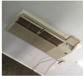
2 604 Unit 604-02 Other - HVAC
