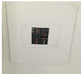
31 612 Unit 612-27 Other - Breaker Box
