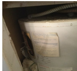
32 612 Unit 612-27 Other - Water Heater
