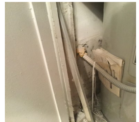
25 612 Unit 612-22 Other - Water Heater
