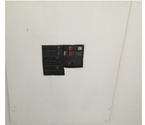
29 612 Unit 612-25 Other - Breaker Box
