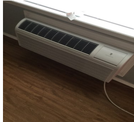
27 612 Unit 612-24 Other - HVAC
