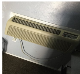
12 608 Unit 608-13 Other - HVAC
