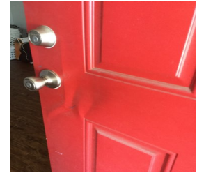
4 604 Unit 604-07 Entire Unit - Front Door/Door Jamb
