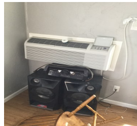
24 612 Unit 612-21 Other - HVAC
