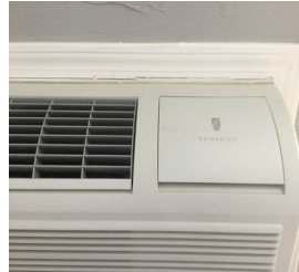
28 612 Unit 612-25 Other - HVAC
