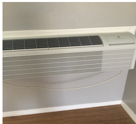
30 612 Unit 612-26 Other - HVAC
